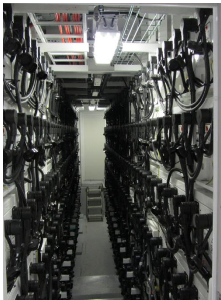
Installation of a 399 x 6.5 kWh battery plant
